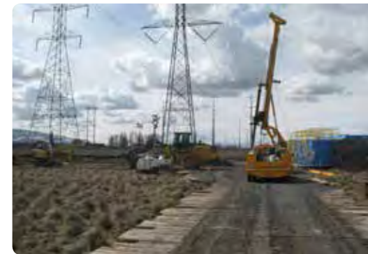
Local Project Success: Legacy Utility Line Construction Removable roadway placed on ground to facilitate access for large equipment so damage to site is minimized. Photograph by Eric McCulley
